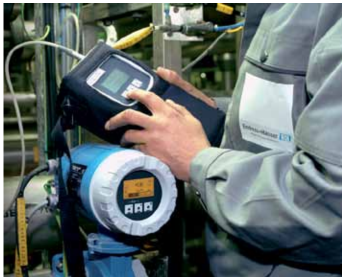
Figure 7. On-site flow verification performed with a test and simulation device - removal of the instrument from the pipe is not required.
