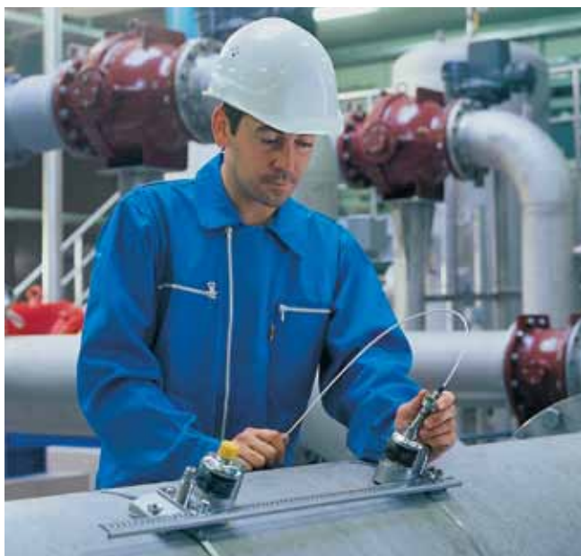
Figure 8. Clamp-on ultrasonic flowmeter used to check flowmeter's operation.
